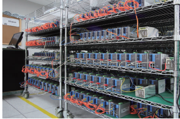
Real-world testing of Turbo Chain with 250 EDS switches
